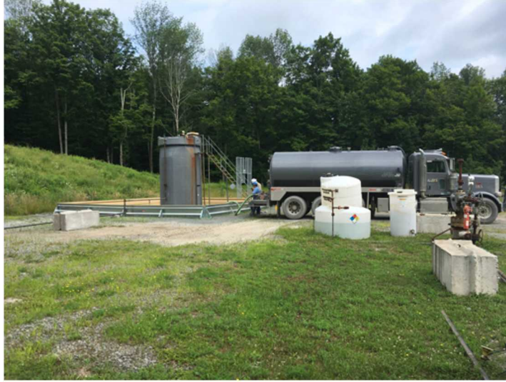
Photo #3. GDS truck actually arrived on location to remove accumulated rain water from secondary containment around Production tank.
